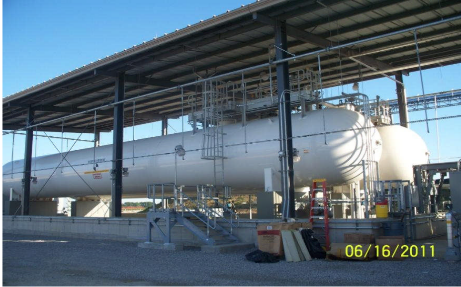
Ammonia Storage System
