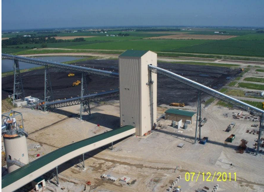
Coal handling and storage area at Power Plant
