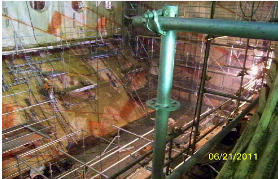
Inside the Unit 2 Furnace
